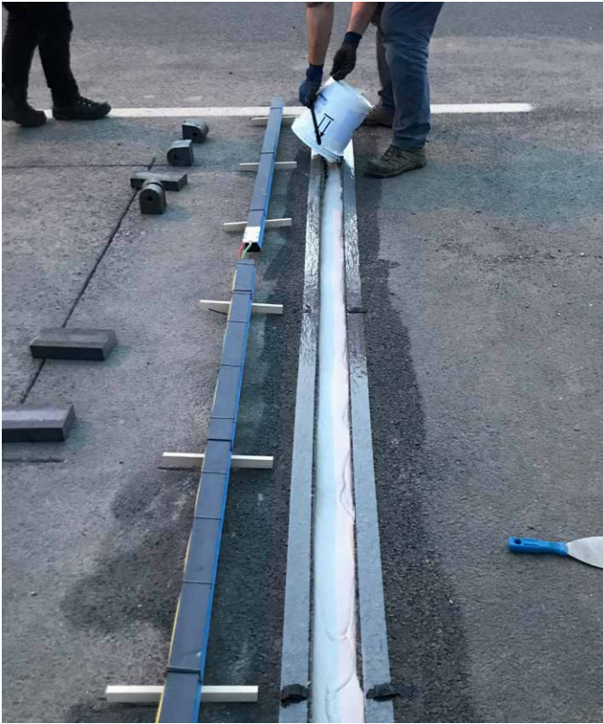
Before the Kistler Linesas WIM sensor is installed, the slot has to be filled with a grouting compound. This is a 3-component epoxy resin composition, specially developed for this installation.
