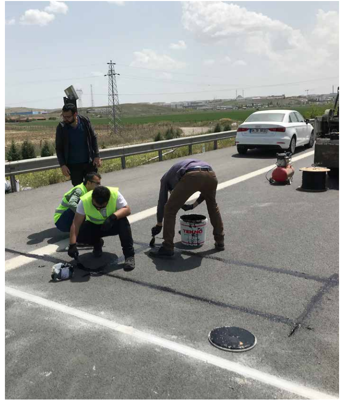
The grouting compound ensures a smooth road surface above the Kistler Linesas WIM sensors.
